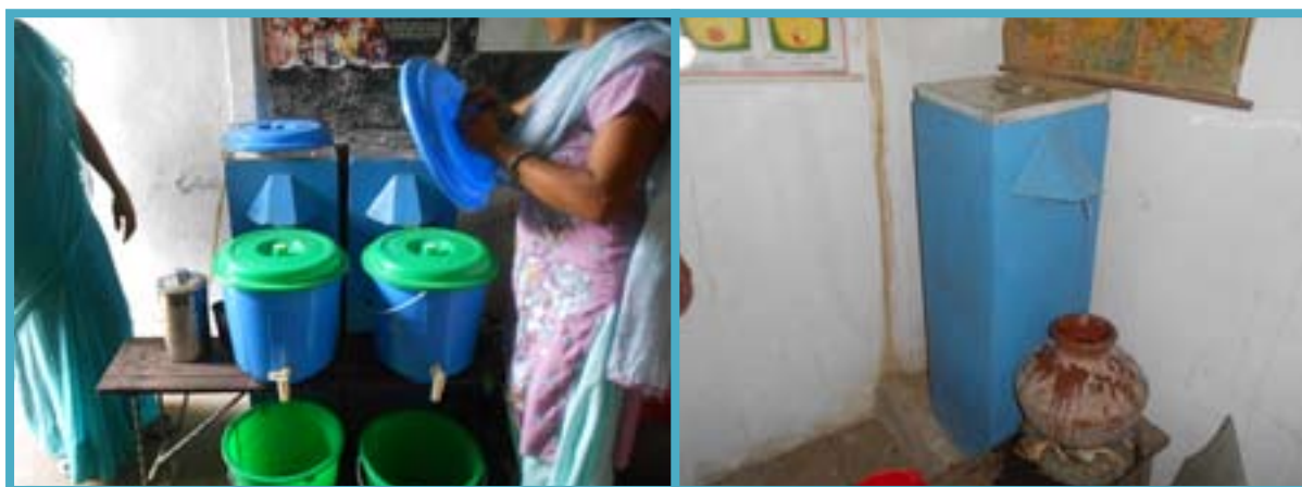
BSF and collection tank: In good condition and covered properly (left); operated after re-installation by the mason with uncovered collection pot (right)
