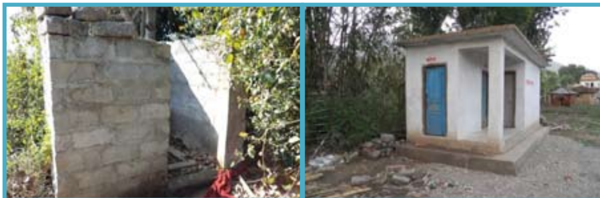
Public toilet construction at Mehelkuna VDC: Before and after new/re-construction (left to right)
