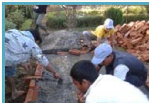
Construction of ECOSAN toilets during the refresher training for masons at Birendranagar in Dec 2013.
