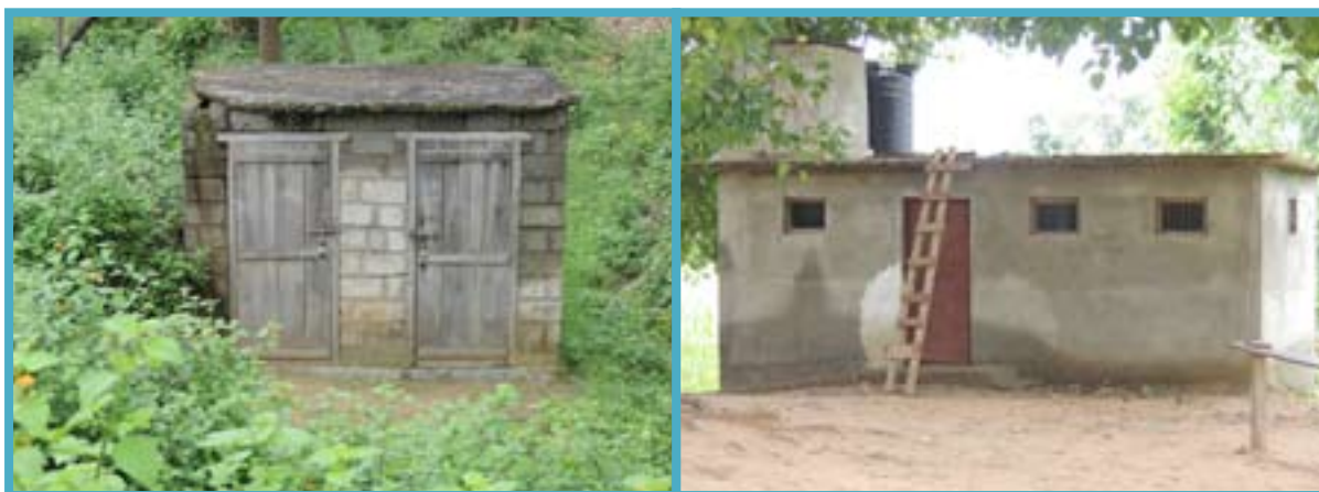
Latrine rehabilitation, Source protection, child-friendly hand washing platform and water supply pipeline installation at Nepal Rastriya NMV, Mehelkuna-8. Before intervention (left) and after intervention (right)
