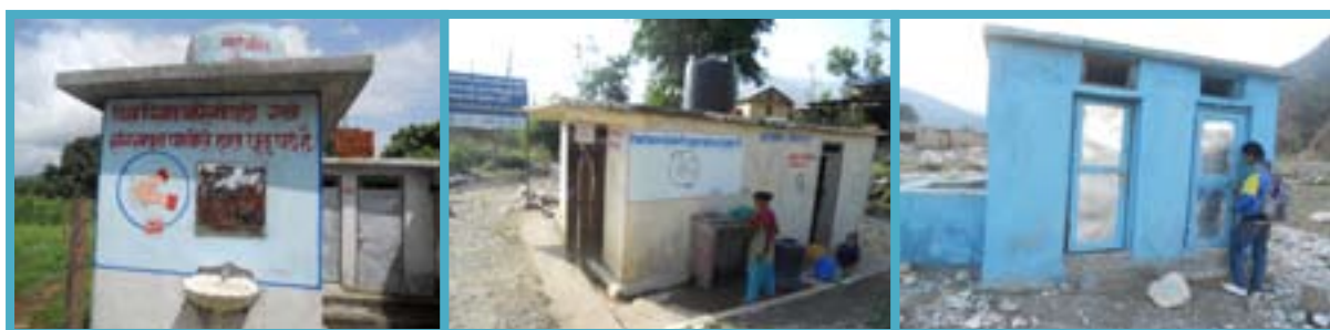
Public toilet construction at Ramghat, Sahare and Kaprichaur (from left to right)
