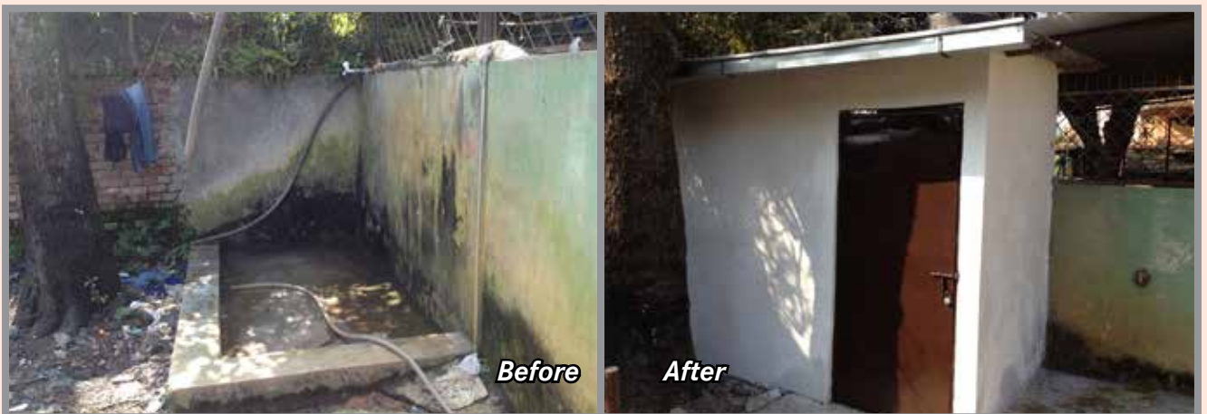
Construction of bathing room and washing platform for hostel children at Central Higher Secondary School for Deaf
