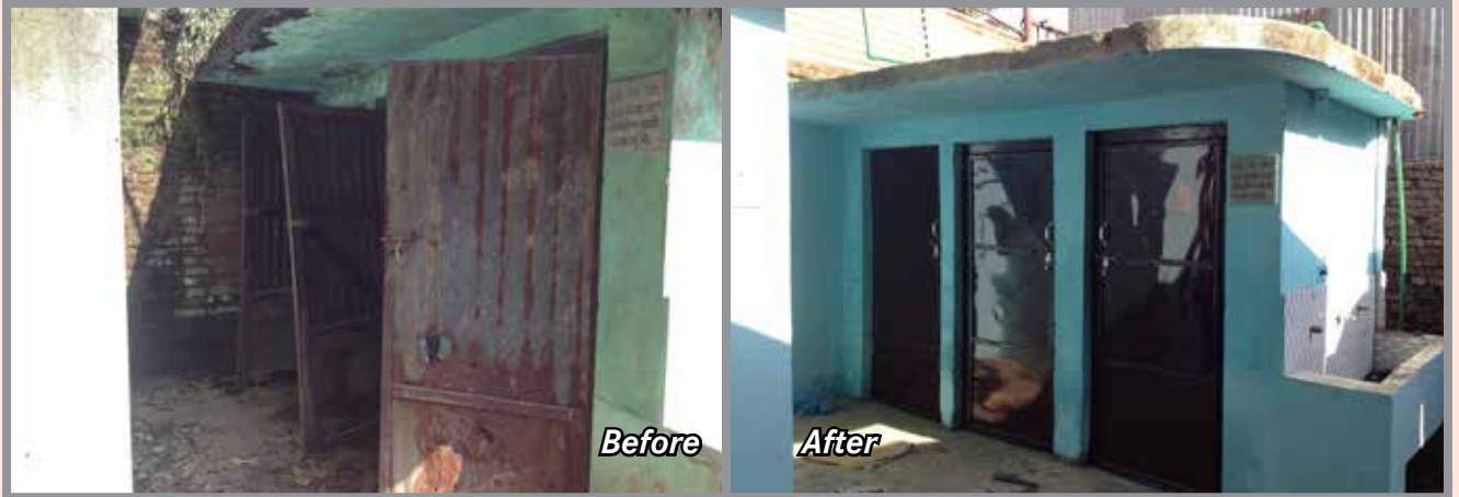
Renovation of toilets and handwashing platform at Mahendra Saraswati Lower Secondary School
