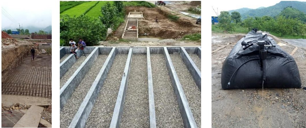
Components of constructed FSTP
