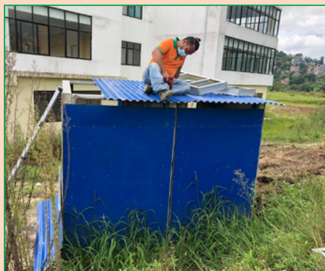
Mr. Shushil Nhemaphuki, Technical Assistant Officer at ENPHO installing toilet at isolation centre in National Ayurvedic Research and Training Center, Kirtipur.
