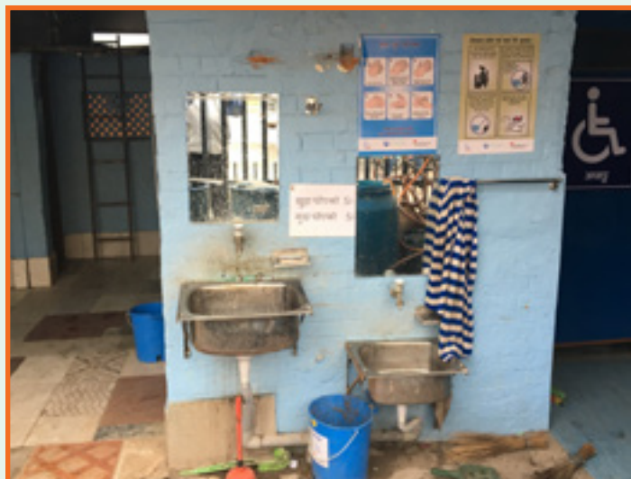
AEROSAN Hub Public Toilet in Ratnapark
